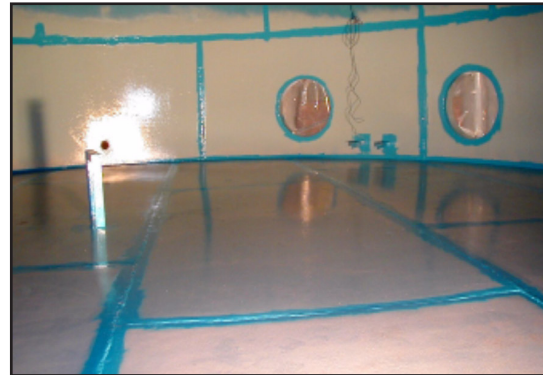
Stripe coating of the weld seams between the first and second coat of ARC S1PW
